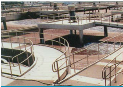
Tubli Pollution Control Center
